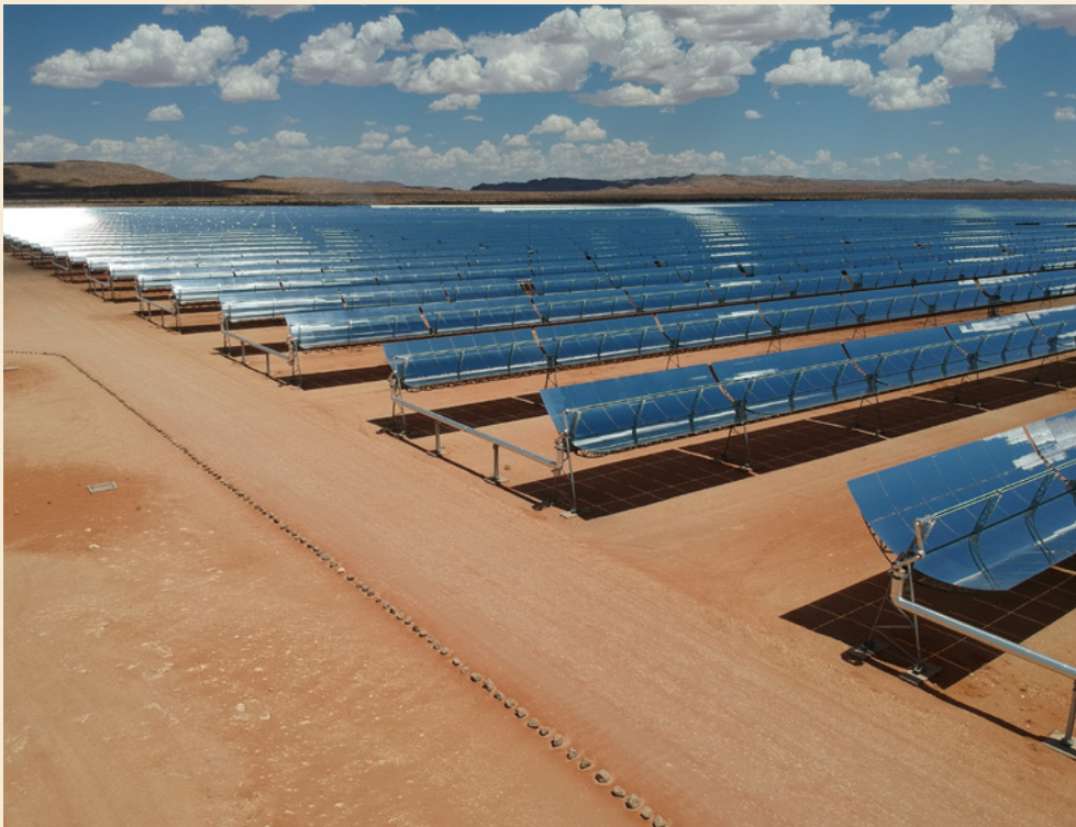
Solar power plant in South Africa.
