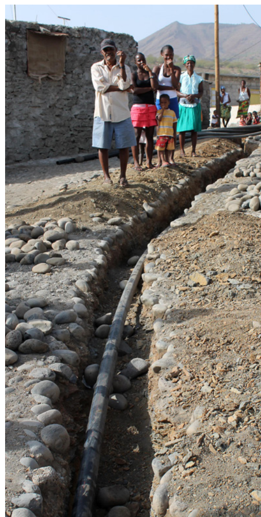
Construction of the first water network of the Communities of Ribeira Grande de Santiago in Cabo Verde, funded by Spanish Cooperation.
